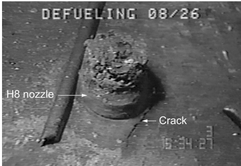
Fig. 2. Photo of the H8 instrumentation nozzle with crack on RPV cladding (Photo courtesy General Public Utilities).
